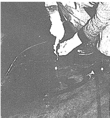
Repairing the concrete. Note discoloration marks left by the water flowing into the liner.
