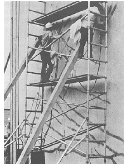
Structural injection resin is injected into cracks through ports made at intervals in the temporary seal. Pumping continues until the liquid adhesive appears at the next immediate port.
