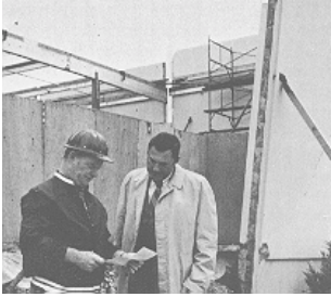
Outside the collapsed Vector building, D. F. Moran (left) consults with his contracting manager, about the application of epoxy injection repairs to the 25 cracked concrete tilt-up panels.
