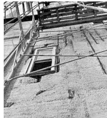
1967. Exterior of Ferry Building prior to guniting. The concrete was 61 years old and showed deterioration caused by rain, moisture and salt air.
